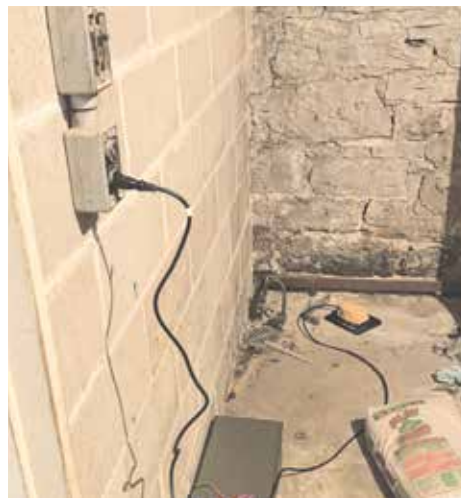
Figure 5. Continuous monitoring of construction vibrations in the building's basement adjacent to a stone wall.
