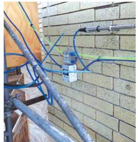
Figure 6. Continuous monitoring of movement across a pre-existing crack in brick masonry façade and overall building movement.
