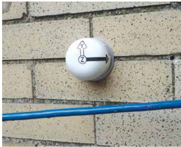
Figure 7. Continuous monitoring of brick façade movement with tiltmeter.
